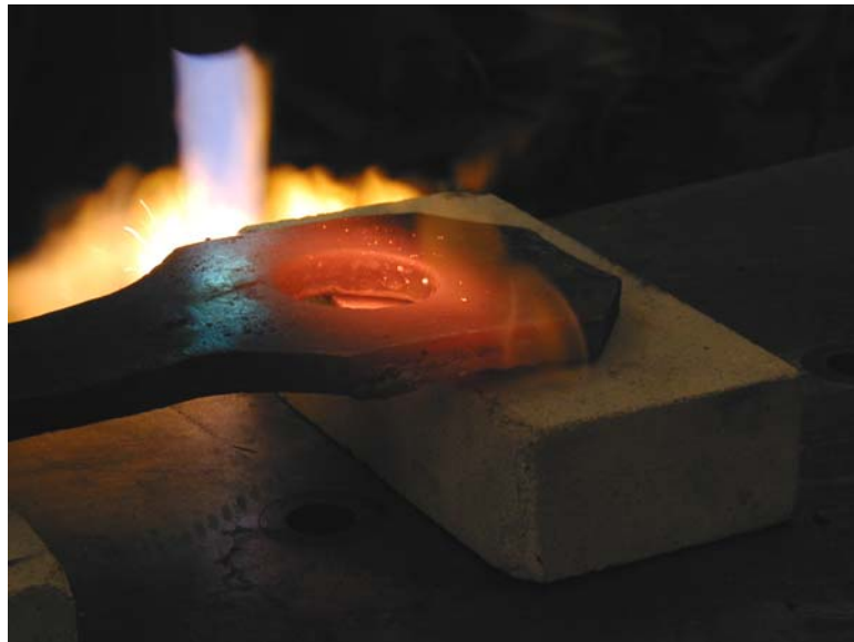
Figure D.10 Heating of Eyebar Connection B to Cherry Red Color before Straightening
