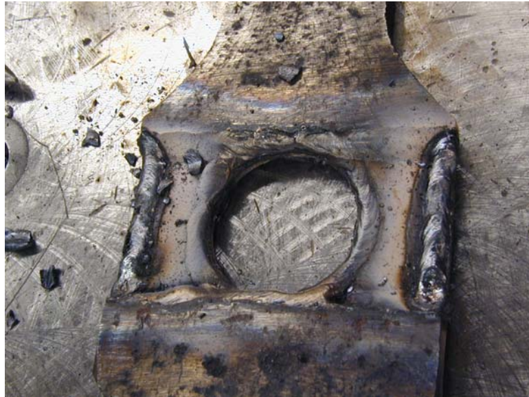
Figure D.7 Initial Pass Pattern on Eyebars B
