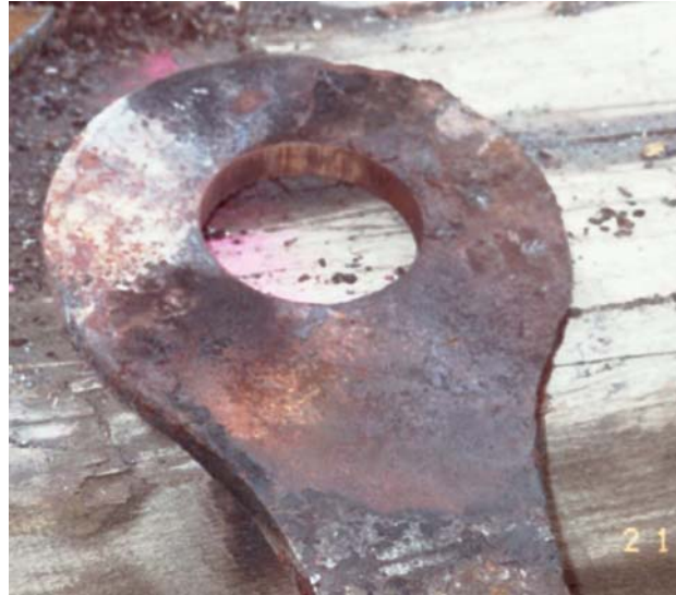
Figure 5.9 Heavy Corrosion in an Eyebar End Connection
