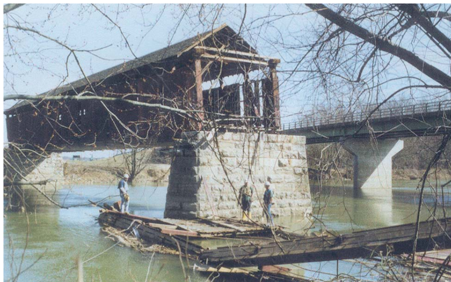
Figure 3.1 Bell Ford Bridge After Collapse of One Span
